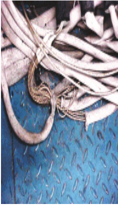
Worn electrical wiring
